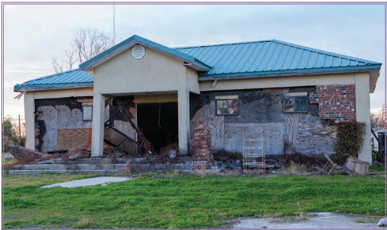
Image 2. Ironton’s only convenience store, which was severely damaged by Hurricane Katrina in 2005
